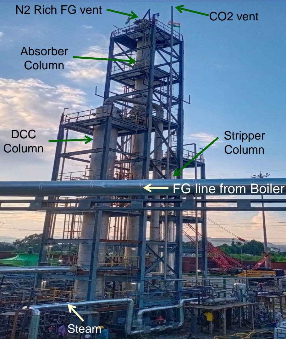
20 TPD CO2 Capture Plant
