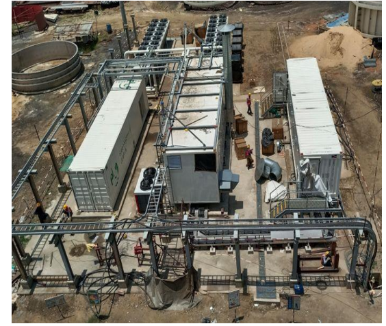
2 TPD PEM H2 Electrolyser Commissioned
