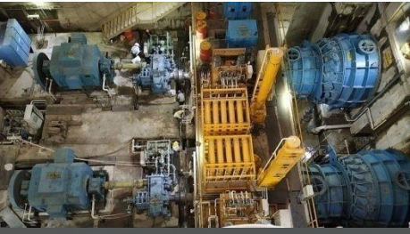
8MW Hydro Plant
