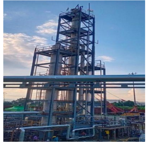
20 TPD CO2 Capture Plant Commissioned
